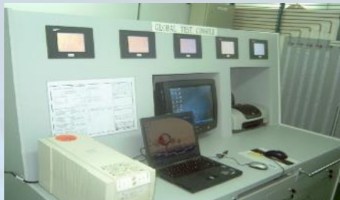
Portable Global Test Control Room – 4 units
