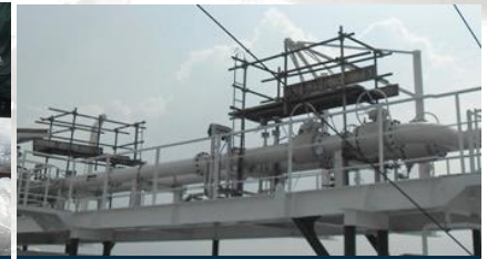
Gas Metering Skid
