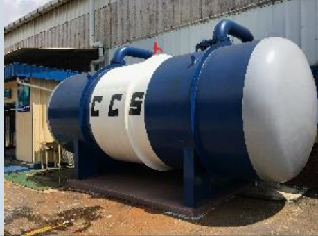
Dry-Air Tank Facility for Cryogenic Safety Valve
