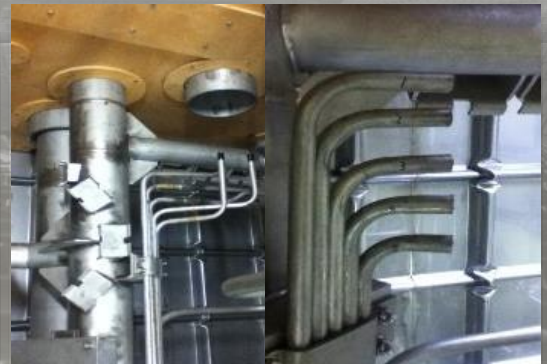
CTMS Upgrading (Capacitance to Radar)
