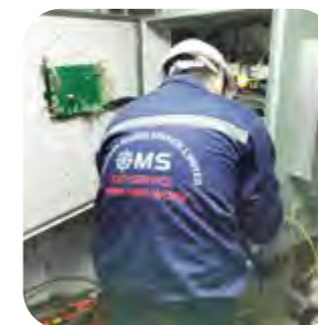
INSPECTION ICCP POWER UNIT
