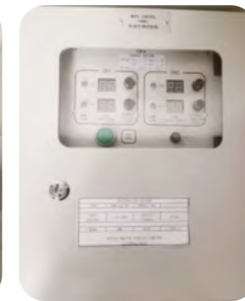
MGPS POWER CONTROL UNIT
