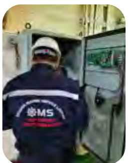
INSPECTION ICCP POWER UNIT
