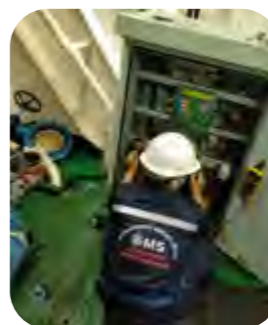
INSPECTION ICCP POWER UNIT
